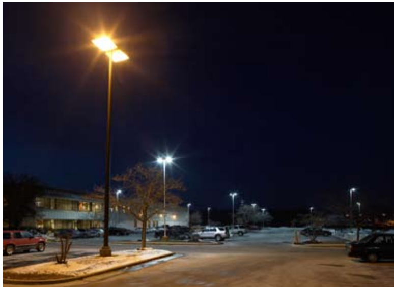
GE Healthcare chose the bright white Ruud LED fixtures (background) to replace the yellow tone of the more traditional High Pressure Sodium (foreground)
